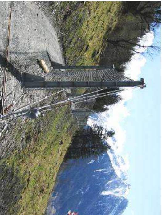
500kJ Rockfall Barrier without upslope anchors positioned near a maintenance road
